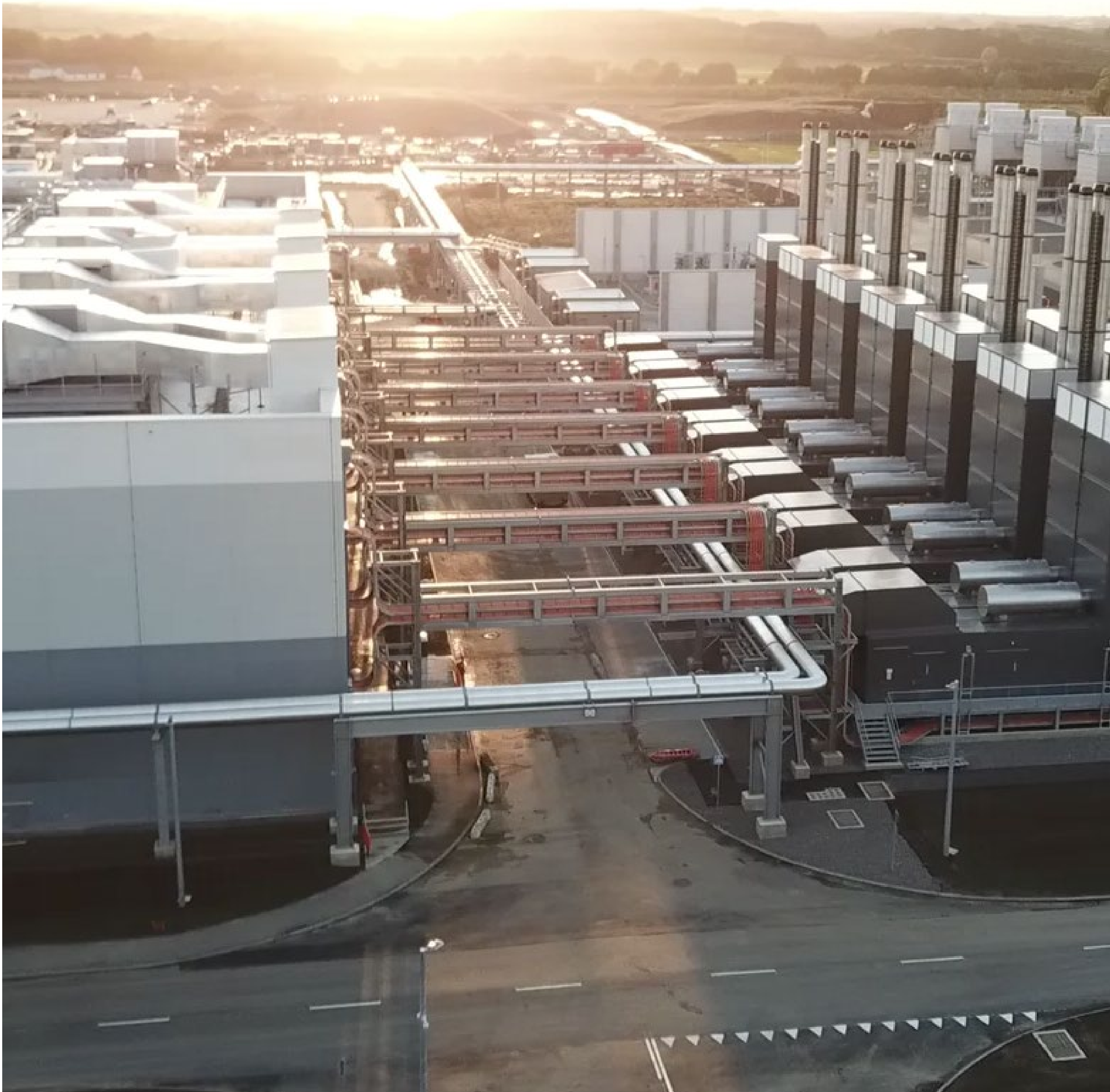
FREDERICIA DATA CENTRE, DENMARK
